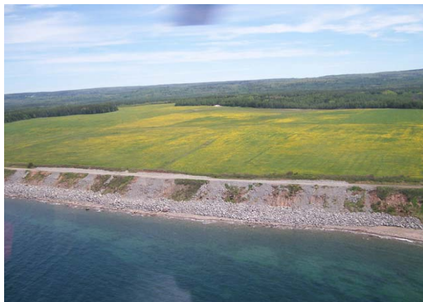
Aerial view showing the beauty of the trail but also the challenges due to coastal erosion.
